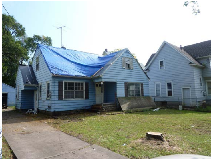
Above is 768 Eagle Street, Dunkirk before CCLBC intervention.
